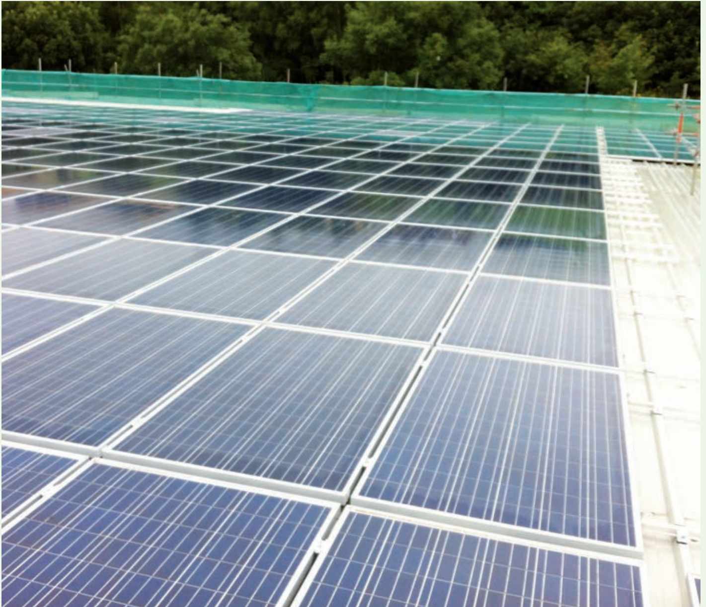
Cold store 250 kWp
